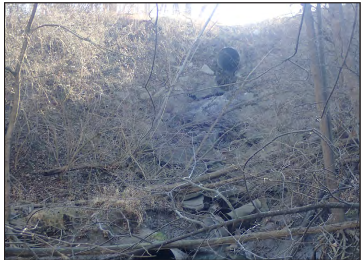
Broken and eroding storm sewer outfall in the western portion of the site
